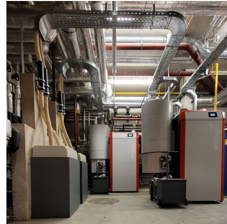
Two 100kW pellet boilers
